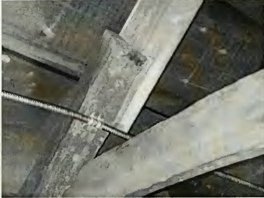
Figure 9 Cut-off Rafter in Center Section of the Main House
